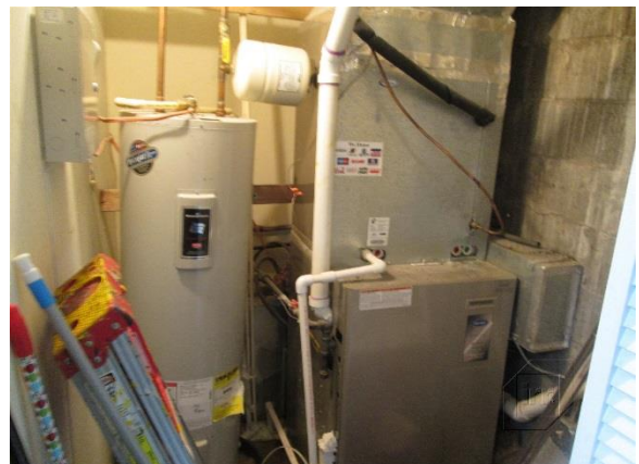
Commercial (Retail) Unit HVAC and Hot Water Heater (Photo Taken on May 2, 2016)
