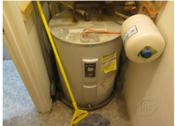
Typical Unit Hot Water Heater (Photo Taken on May 2, 2016)
